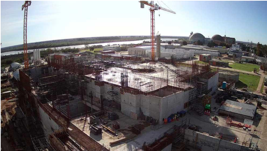
Figure 7. Photo of the progress in the construction of the CAREM project in the Atucha complex
